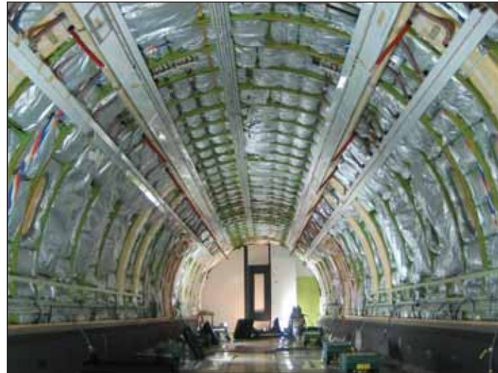
Noise reduction application (by A.I.M.S. Int'l) on a Challenger 870 pending final delivery to customer.
